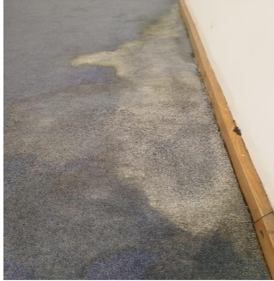
Fig 3b : Our landlord kept promising us for the repair but never seen him
