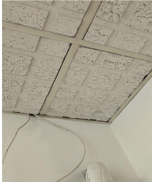
Fig 3a : “Our landlord kept promising us for the repair but never seen him”
