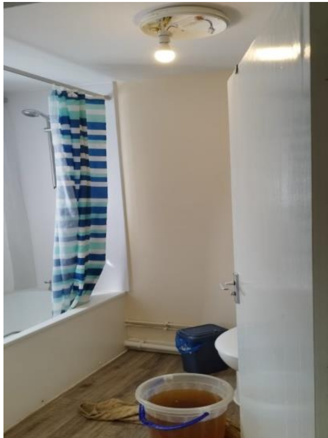
Fig 2 : A safety and health concern where the ceiling is leaking around the lamp holder at the social housing around the Cowley
